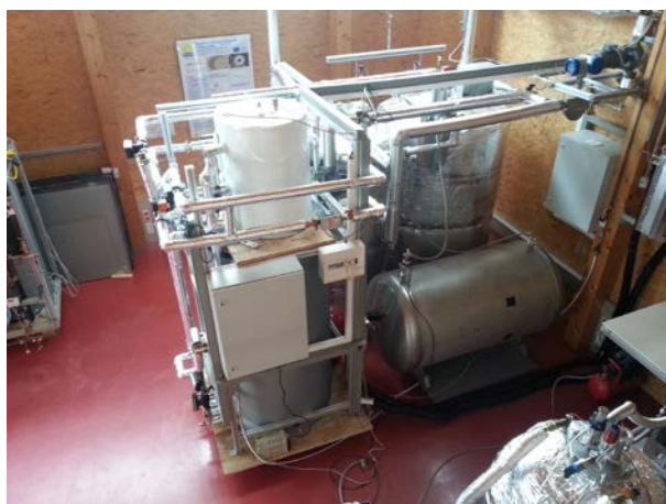
Experimental setup on seasonal heat storage at the AEE INTEC laboratory for EU project COMTES
